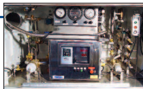
HL Series controls and plumbing
