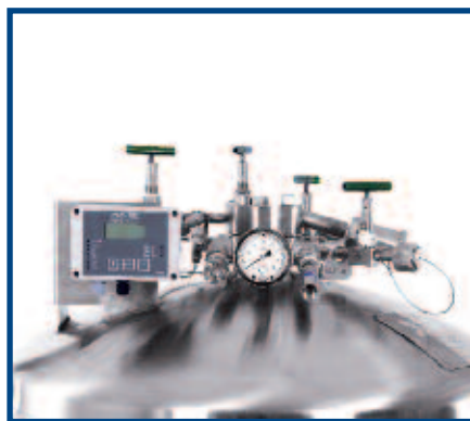
UHP-Stainless steel plumbing for high purity applications
